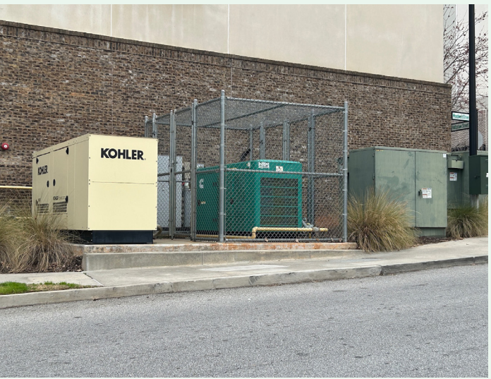
Placement of mechanical equipment between the building and street, along with lack of screening, detract from the public realm.
