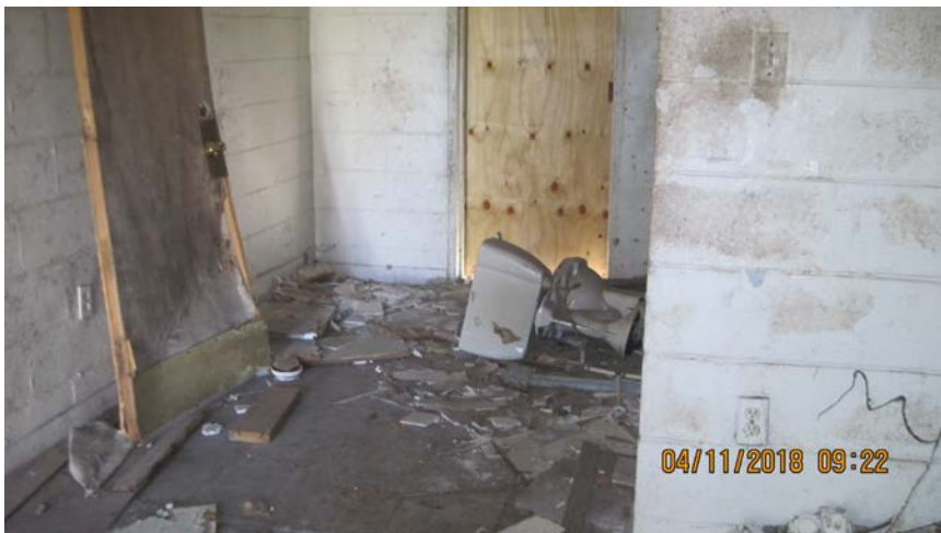
Photo #5 - Interior of one of the vacant apartment units at 800 South Tampa Avenue
