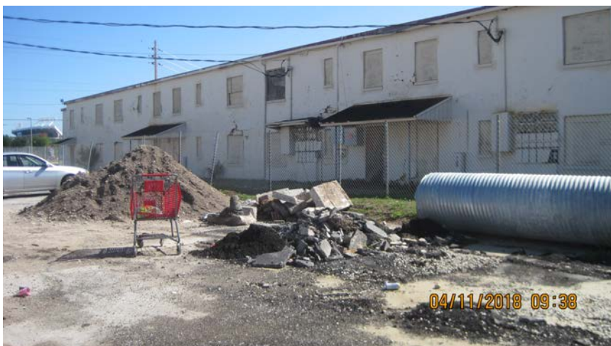
Photo #6 - Rear of vacant apartment building at 800 South Tampa Avenue
