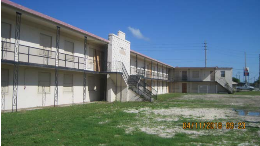
Photo #4 - Front of vacant apartment building at 800 South Tampa Avenue
